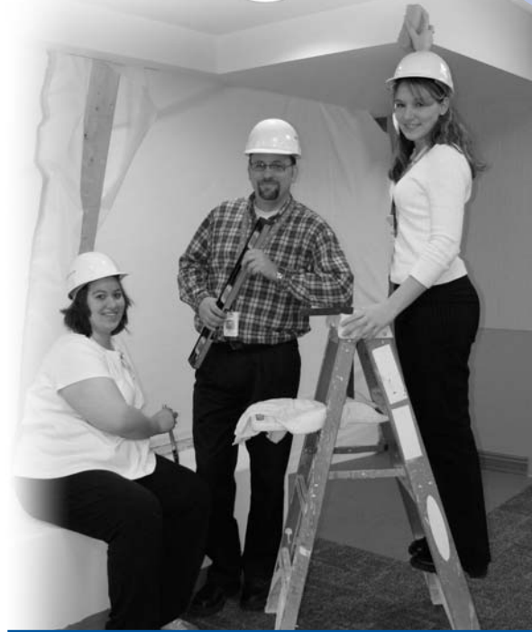
The Morgans' gift will be used to construct the Physical Rehabilitation Education Classroom. Pictured above in the area that is currently under construction are St. Luke's Physical Rehabilitation associates (from left) Amanda Krogmann, James Pazour and Shannon Eck.
